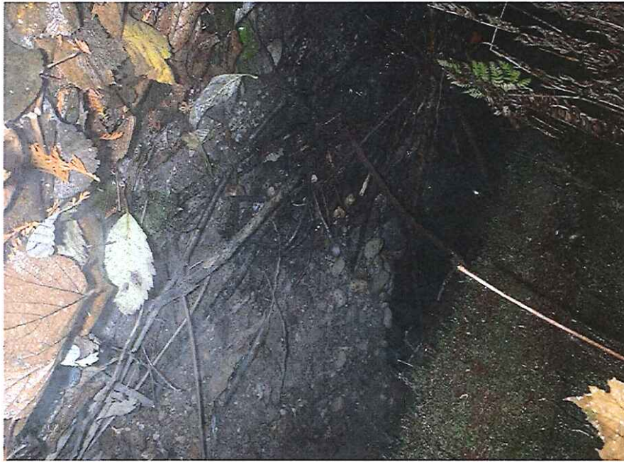
CK2338 Failed fill inside Outlet
