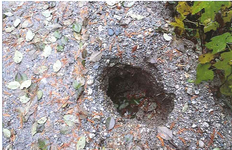
CK2338 Deck hole
